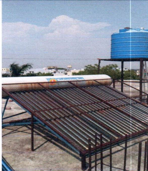
Solar water heater
